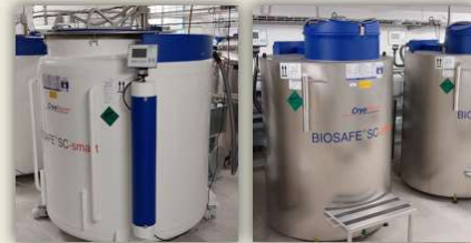
New LN2 tanks
