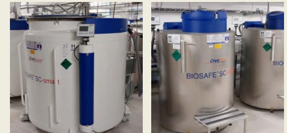
New LN2 tanks
